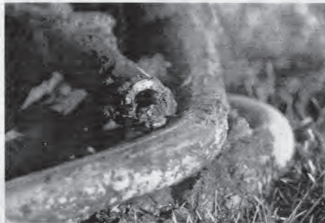
Old lead piping can be seen after removal from a home in Galesburg, Illinois, on March 4. JOSE M. OSORIO/CHICAGO TRIBUNE
